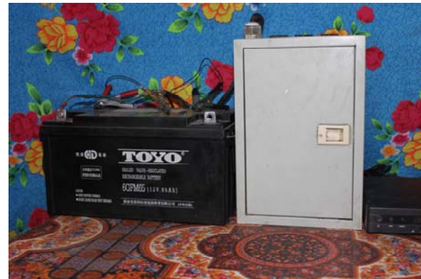
Battery and controller for solar home system
