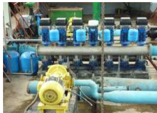
The Boryspil water and sanitation utility upgraded its equipment with a Bank loan.
