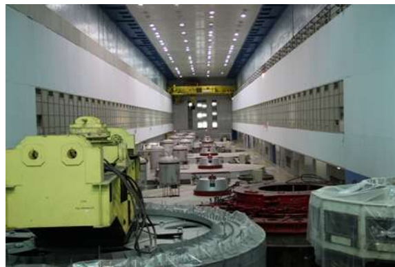
Upgraded hydropower units at the Dniester hydropower plant
